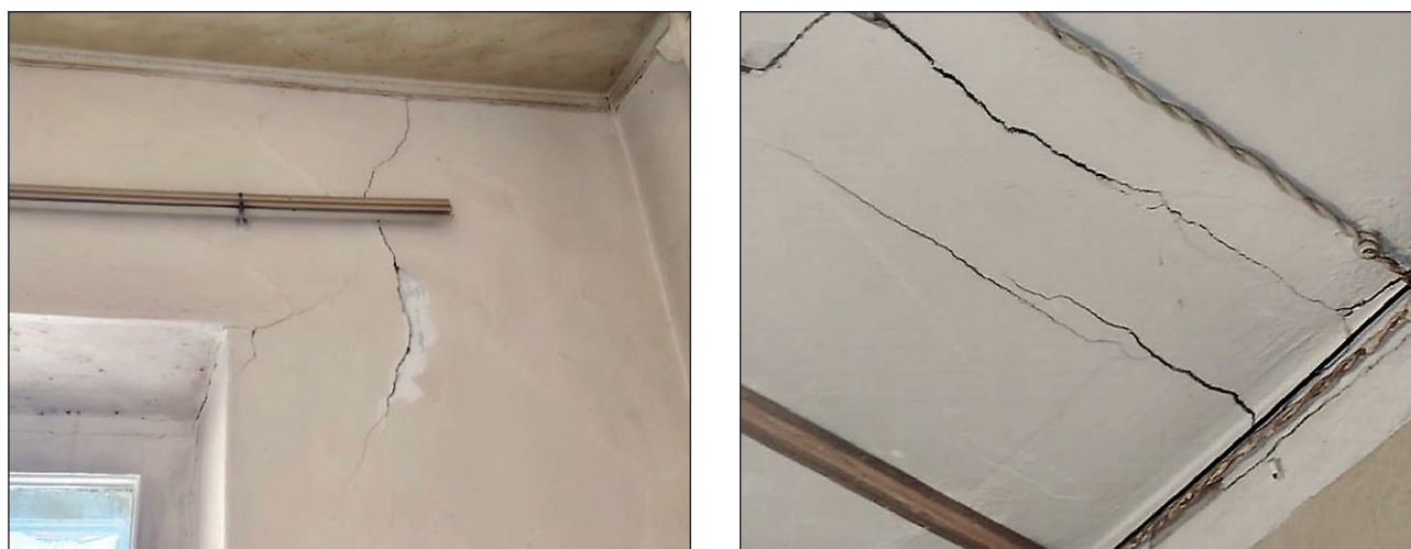
Fig. 1. A building with settlement exceeding regulatory limits (deterioration of the soil foundation, impact of new construction near the building). Vertically sloping cracks on the walls, longitudinal cracks in the floor slabs
