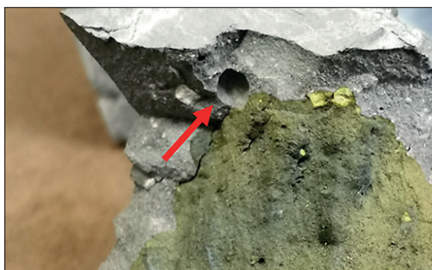
Fig. 1. Crystallization of side reaction byproducts in the pores of concrete. Cracks inside the sample
